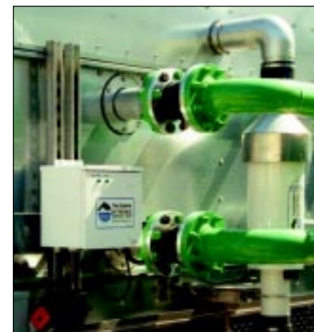
One of 16 Dolphin System Applications on Cooling Towers at a Peaker Power Plant
