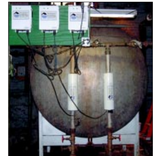
Dolphin System Applications on a Steam Boiler
