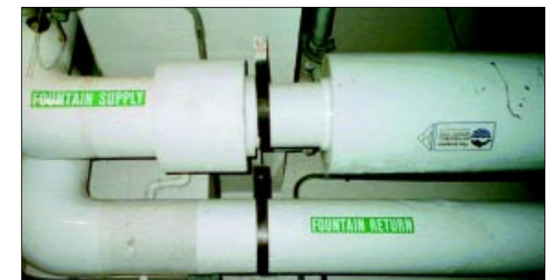
Dolphin System Application on a Large Commercial Building's Decorative Fountain
